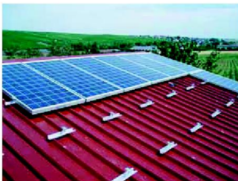
The TRI-VENT support profiles are only riveted to the roof at the points required by the module installation.
